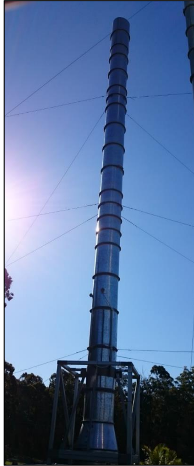
Figure 4-3: EPL Point 3 (Wet Separator Stack)
